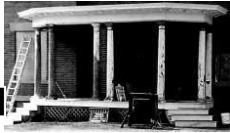
Preserve original porch features. Patch and repair significant features rather than replace.
